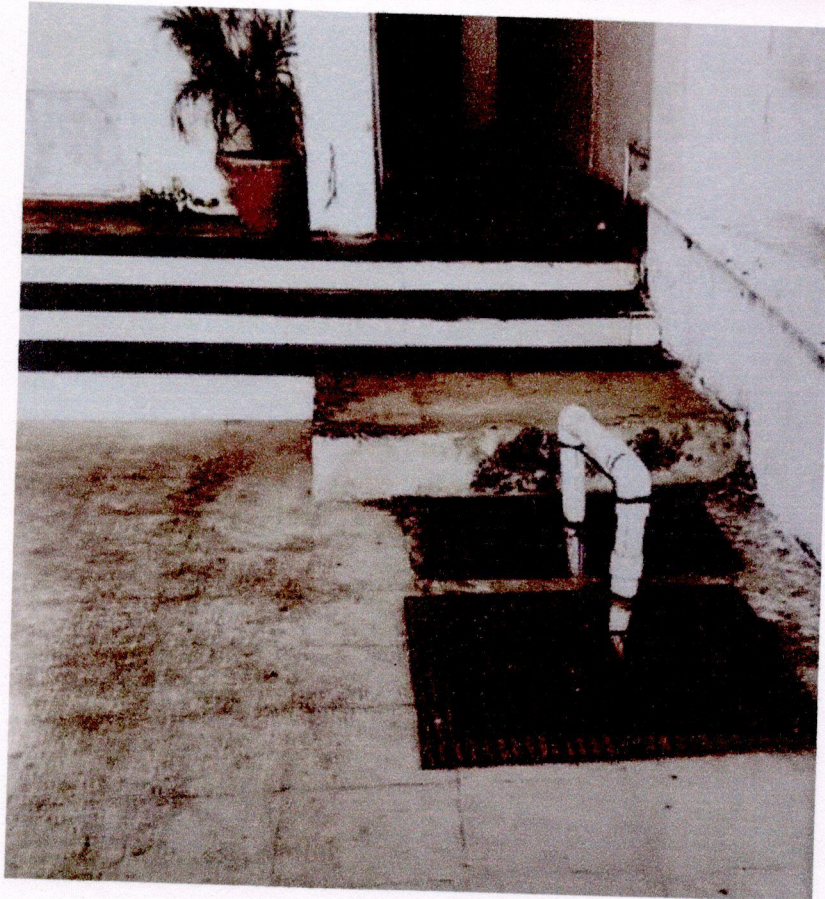
Photo: Tank to Store Rain Water
