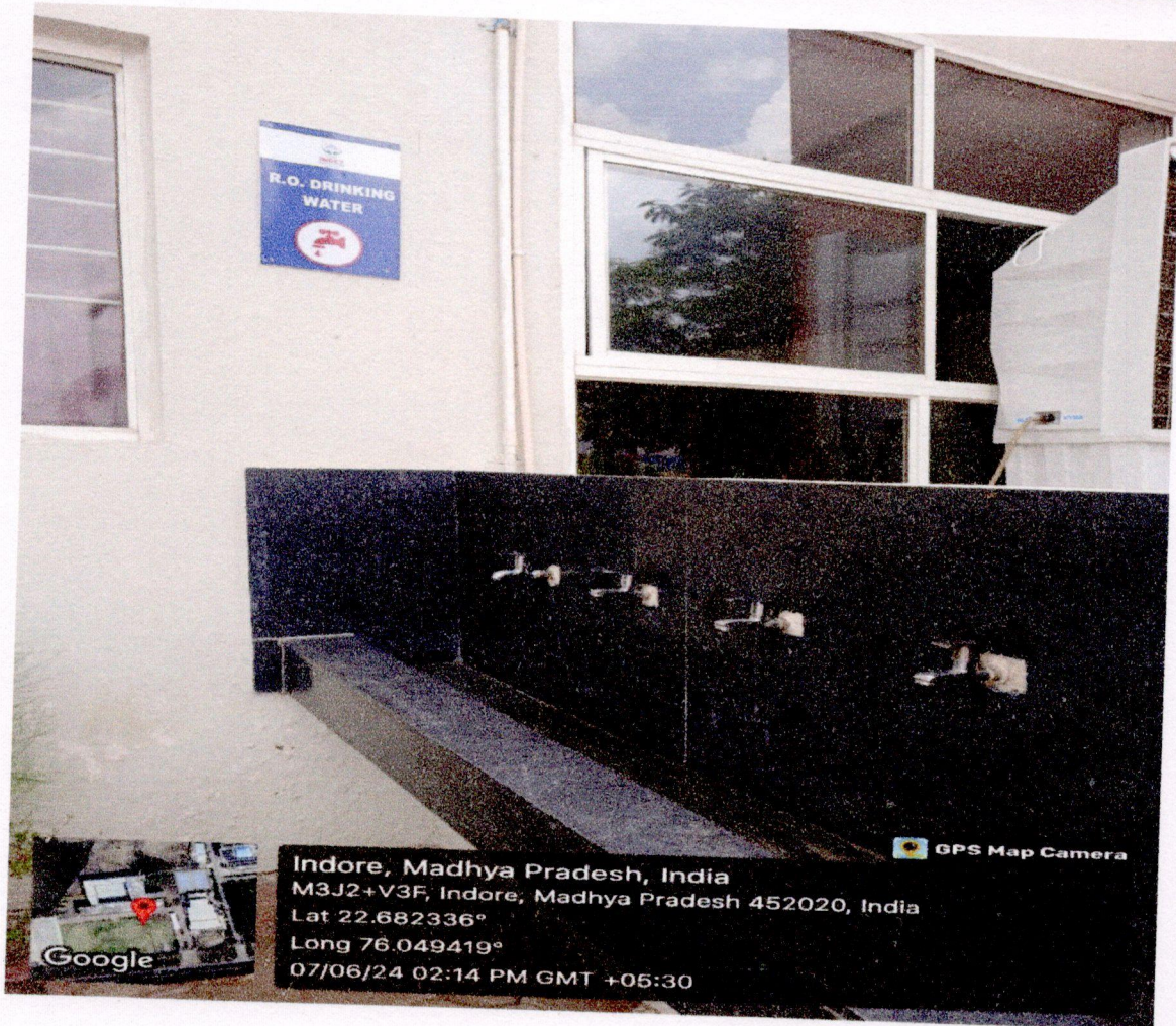
Photo: (RO) Drinking water Facilities
