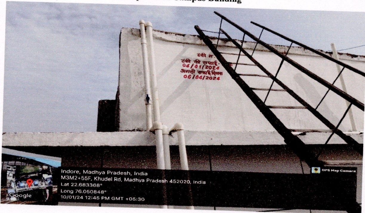
Photo: Over Head Tank in the campus building
