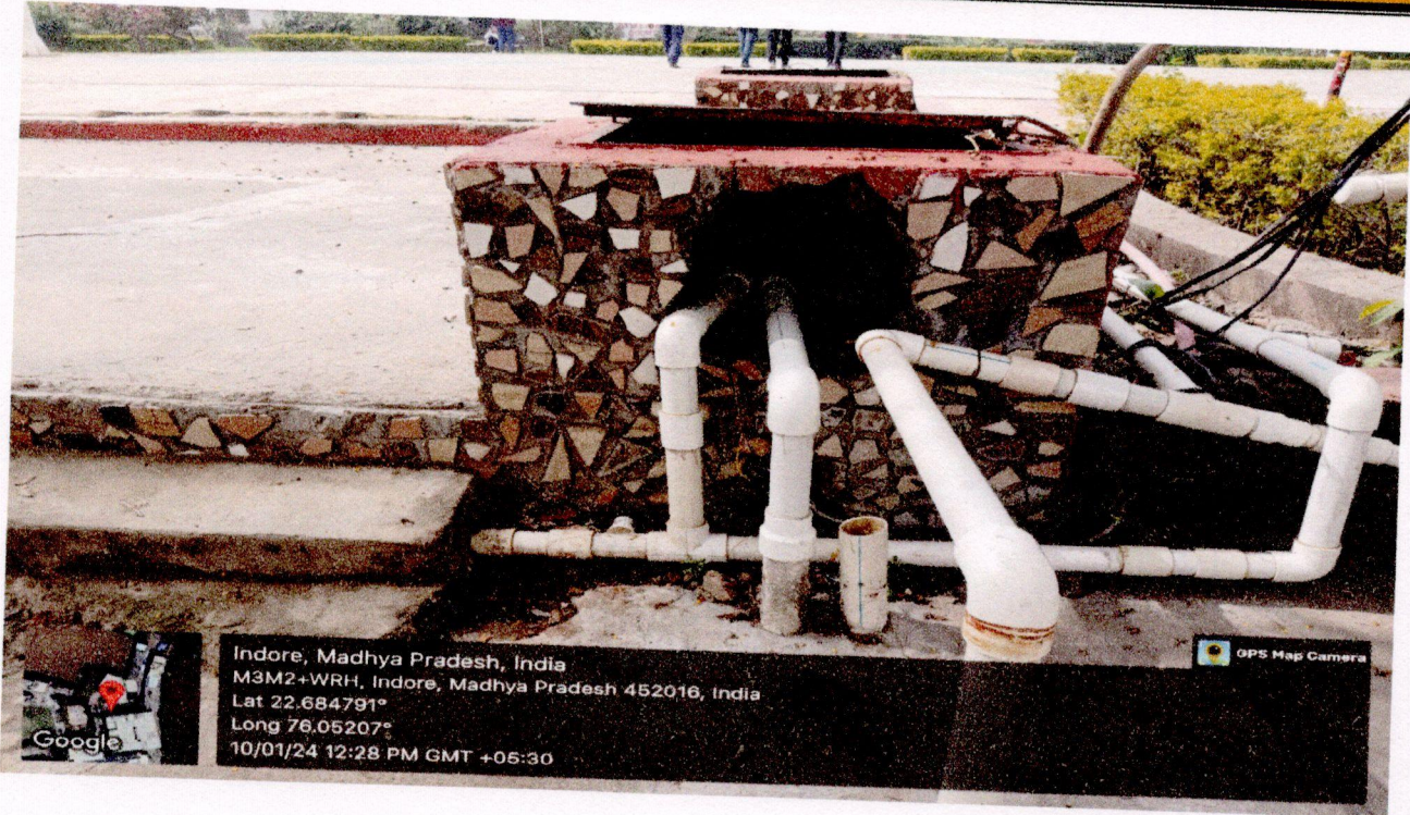
Photo: Underground water Storage Tank in the Campus
